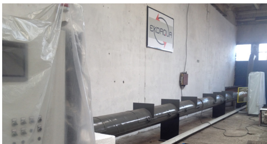
Figure 6. Photo of system on an semi-industrial scale.
