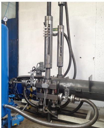
Figure 7. Feeding and compressing system. Industrial scale installation.
